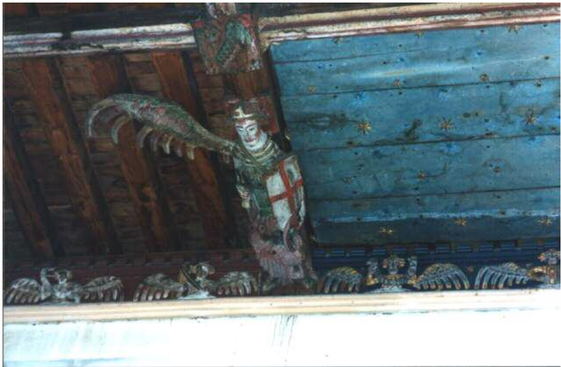
24 St. Andrew, Kimbolton, Cambridgeshire. An Angel with a missing wing in the South Chapel, and small Angels on the wall-plate at his feet.
