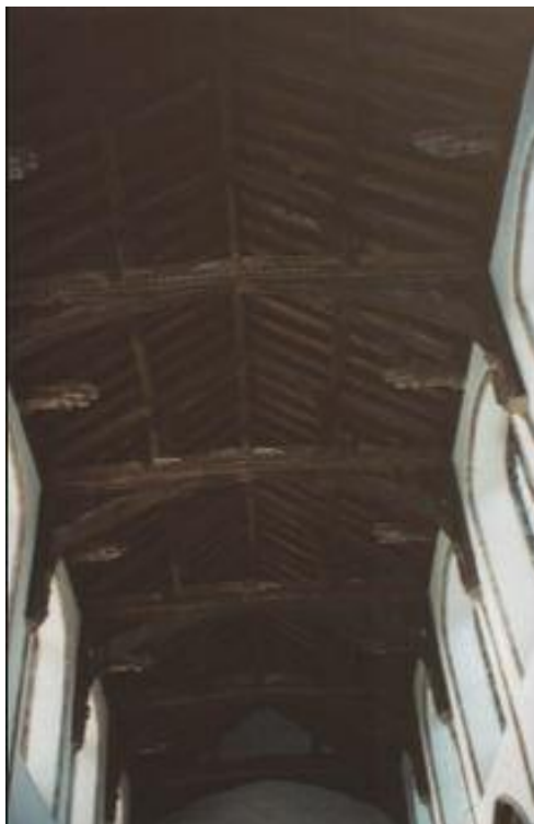
30 St. Edmund, Emneth, Norfolk. An example of an arch braced tie-beam Roof with full-length Angels with folded wings along the sides and demi-Angels with outstretched wings on the tie-beams.
