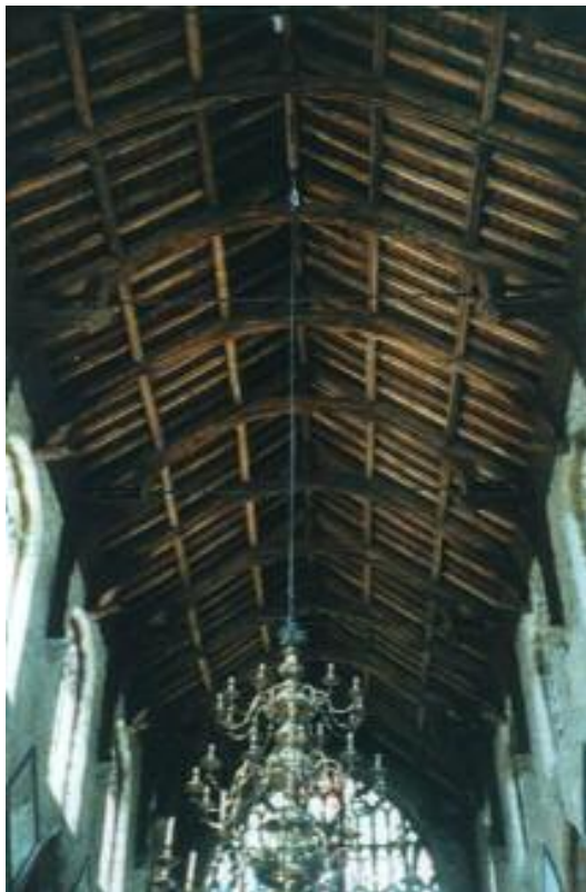
4 St. Mary and St. Nicholas, Spalding, Lincolnshire. View of the iron ties inserted to control the spread of the Nave Roof.
