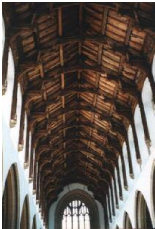
10 St. Peter and St. Paul, Swaffham, Norfolk. View of the Roof showing the span and the double ranks of Angels on the hammers
