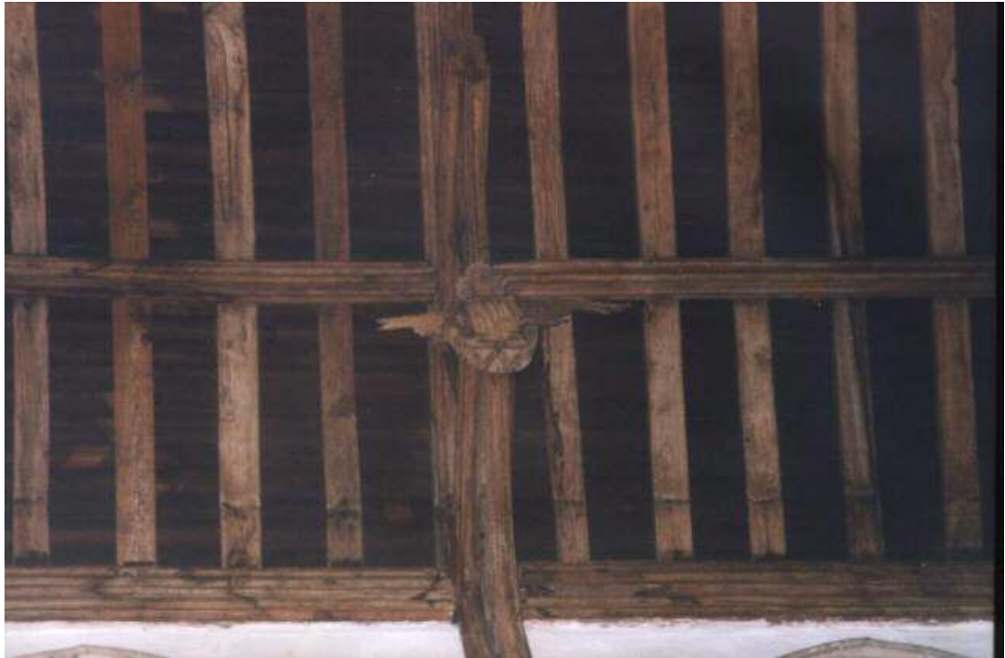
21 All Saints, Elm, Cambridgeshire. Small damaged Angel with broken wings.
