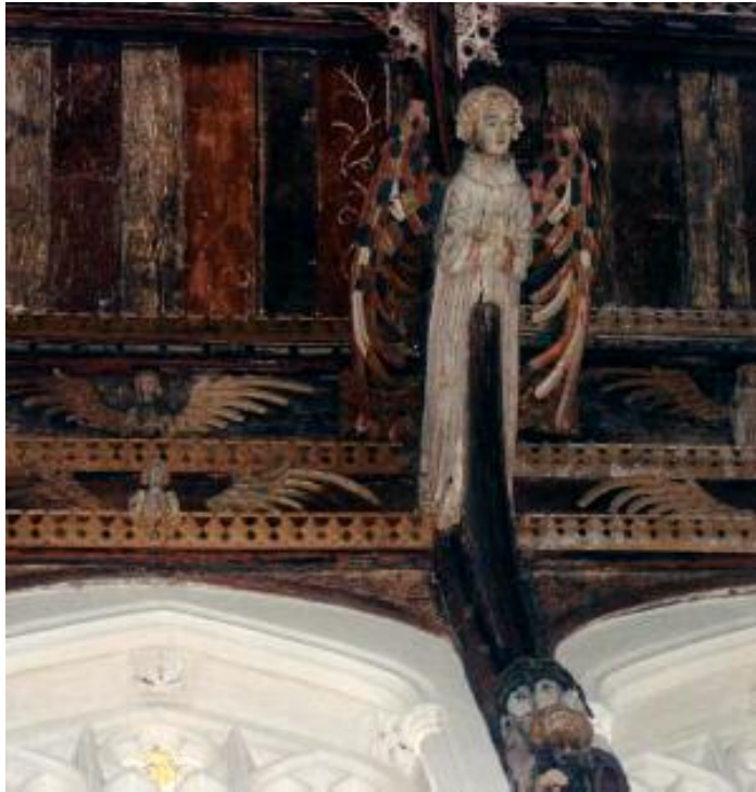
7 All Saints, Necton, Norfolk. The coloured Roof with one of many watchful Angels on the hammers, and a double row of demi-Angels with big outstretched wings on the wall-plates.
